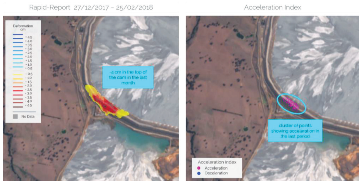
Figure 8. Rapid report and an acceleration index over Cadia mine tailings dam made in back-analysis thanks to archive satellite data a available
